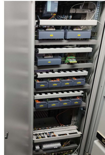
New control rack
