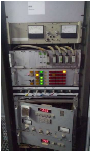
Old control rack
