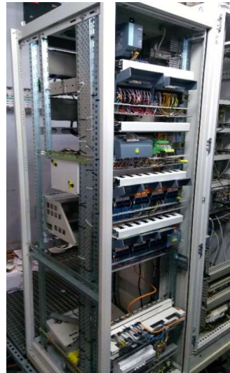
New control rack
